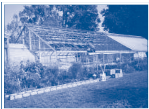
WORKMAN PREPARES FRAME FOR NEW GLASS AS PART OF LAST SUMMER'S GREENHOUSE RESKINNING PROJECT.
